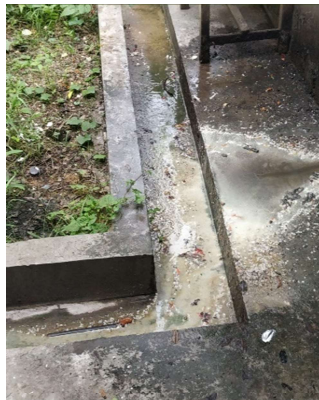
p) Improper use of drainage system in women's hostel
