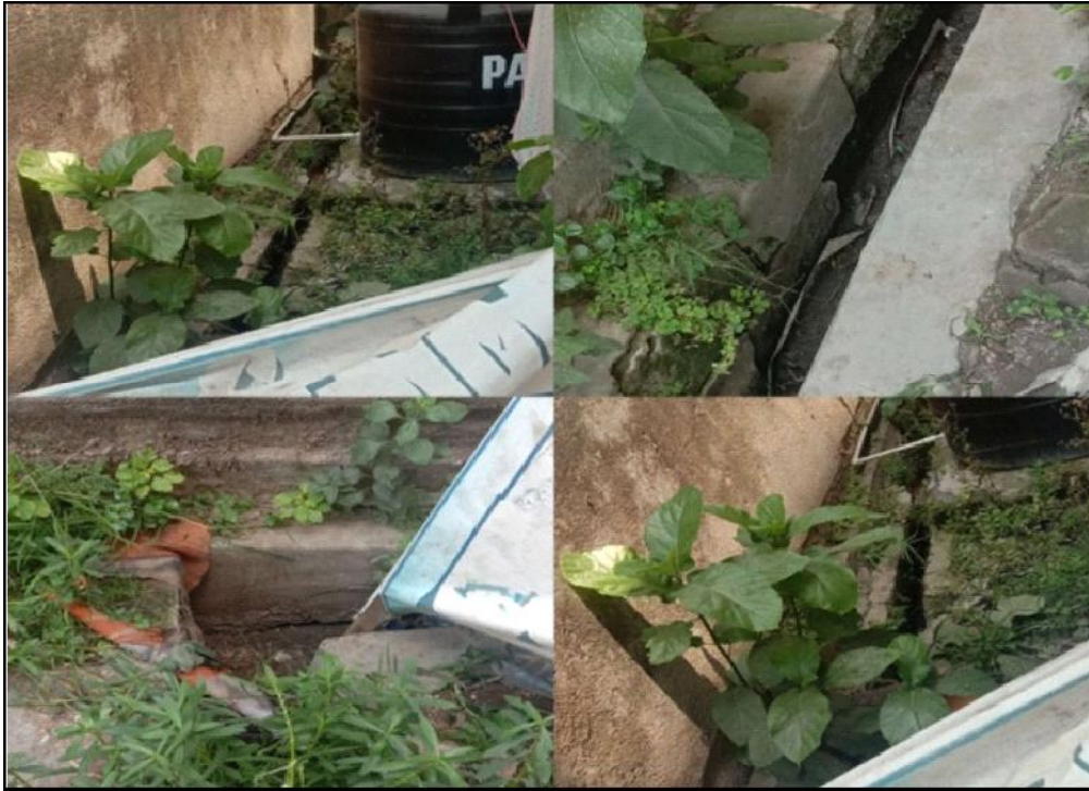
Fig. 8 The drain which runs along our street and it is this common drain where most of the shops and also the households dump their liquid wastes.
